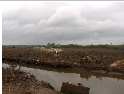
Plate 2: Mangrove vegetation clear-felled in the salt concession area. Note the salt water pipe-line under construction
